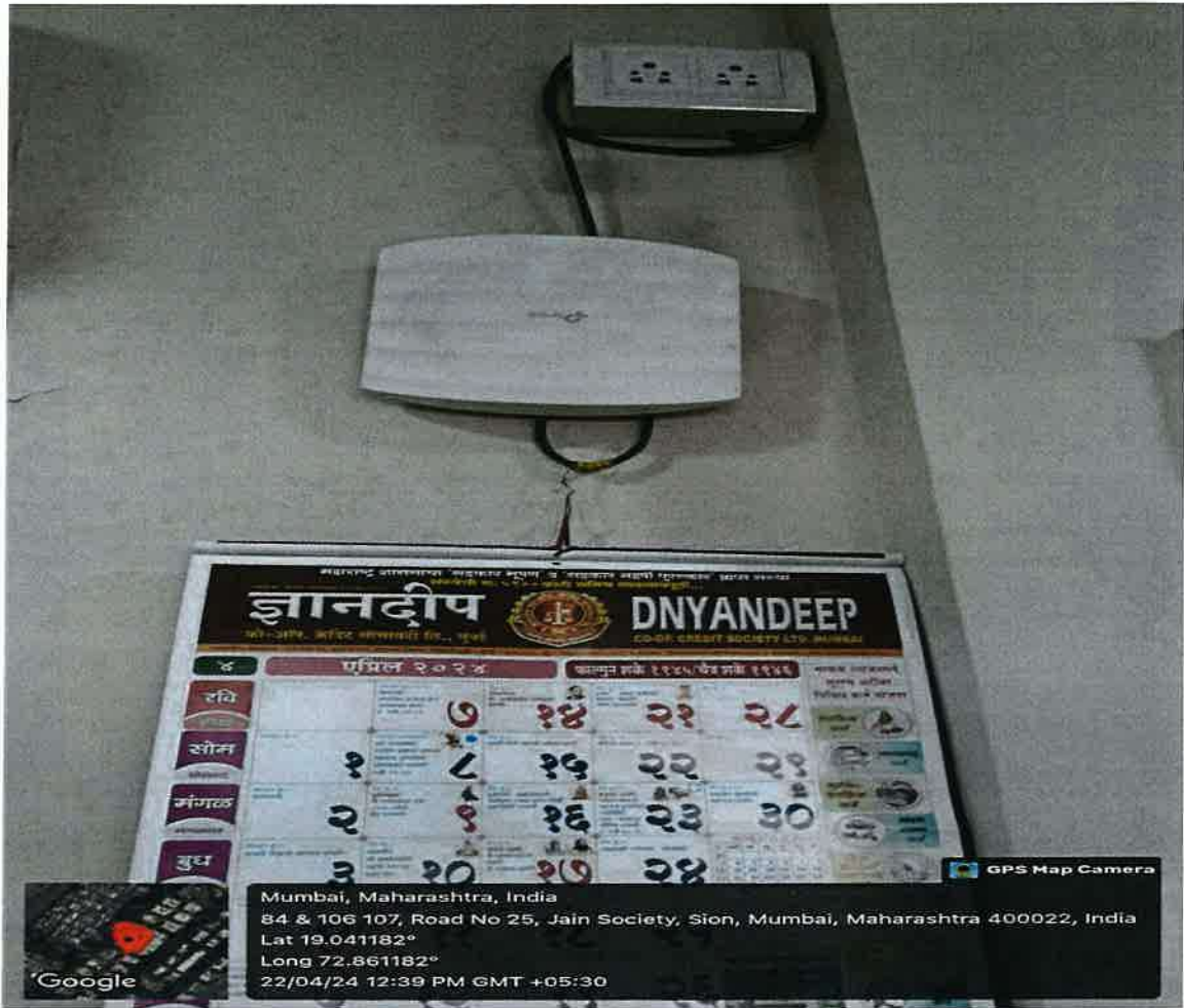
Academic Staff Centre installed since 2018-19.
