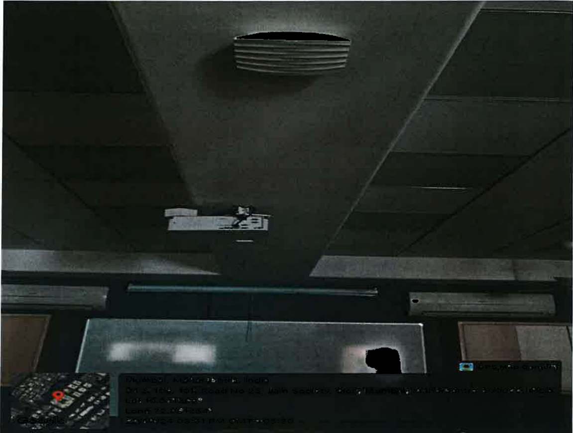
IT Lab – LAB NO 4 - installed since 2018-19.
