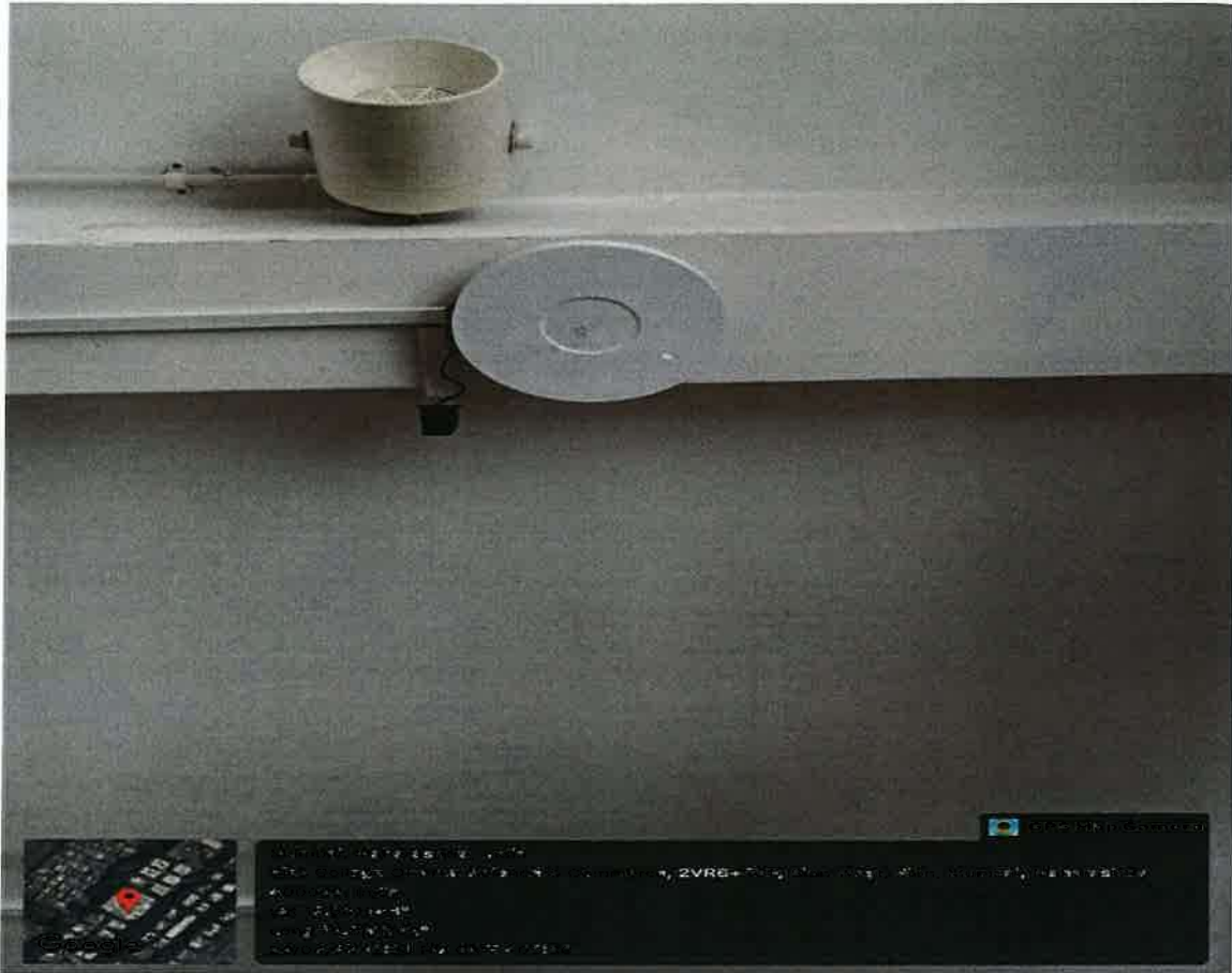
Ground Floor - installed since 2023-24.
